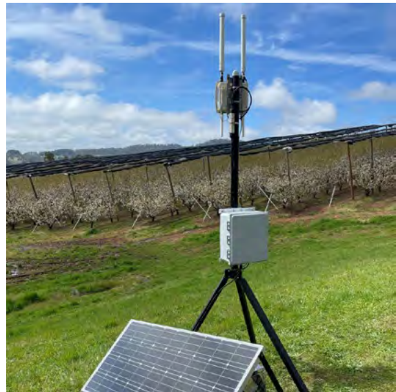
Figure 8. LoRaWAN Gateway (MultiTech Conduit IP67) installed at the Nashdale trial site.
